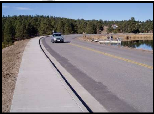
Figure 4 Pedestrian safety was greatly improved with the addition of the sidewalk across Lake Forest Dam.
